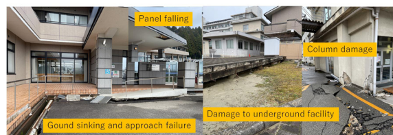
(a) Damage to facilities
