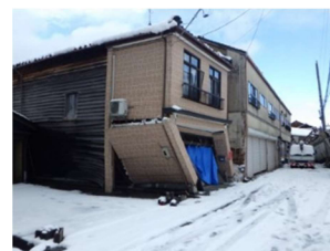
Photo 2-6 Heavily damaged wooden house
