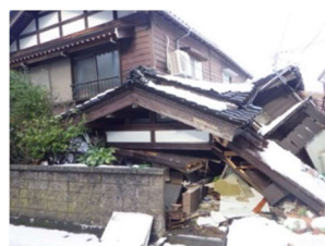
Photo 2-11 Heavily damaged wooden house
