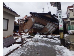
Photo 2-14 Heavily damaged wooden house
