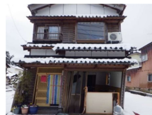
Photo 2-8 Heavily damaged wooden house
