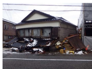
Photo 2-16 Heavily damaged wooden house
