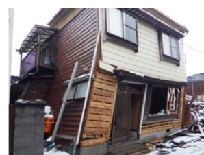
Photo 2-12 Heavily damaged wooden house
