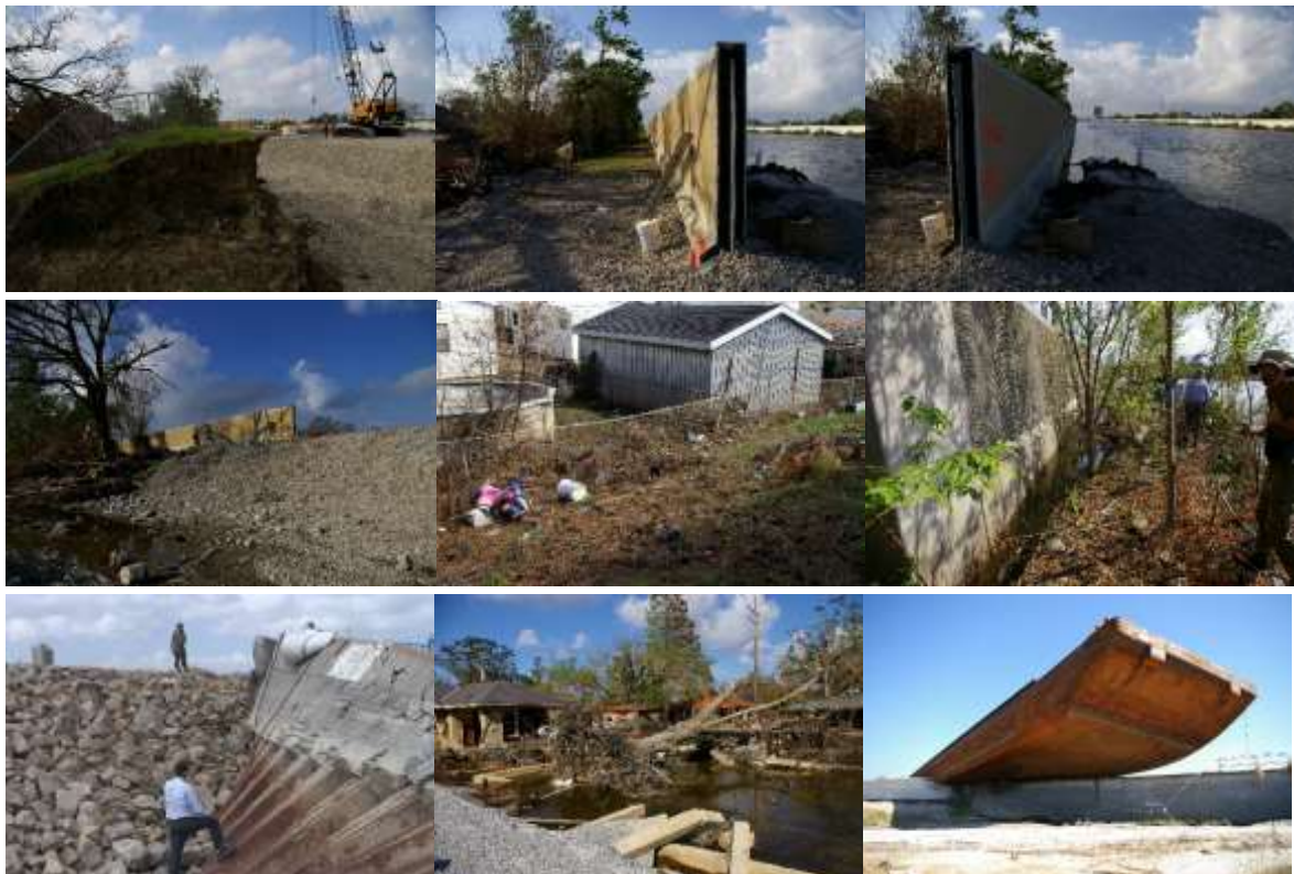
Photo 8 Hurricane Katrina's damages of storm surge protection levee system in New Orleans.
