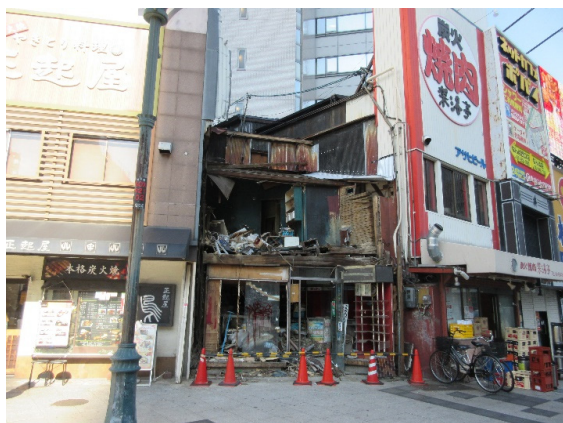
Fig. 2 A damage to an old house
