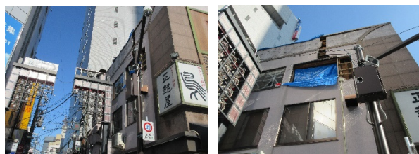
Fig. 3 Damages to houses and buildings
