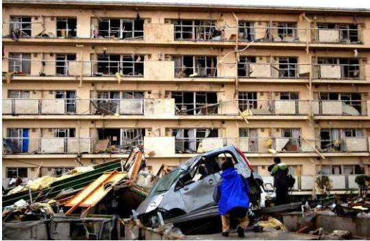
Fig. 9 Damage to five storied apartment house ( quote from the report of KAKENHI, 2013 )
