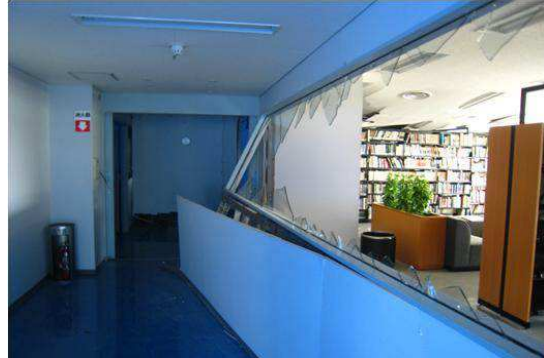
Fig. 10 Damage to interior wall ( quote from the report of KAKENHI, 2013 )
