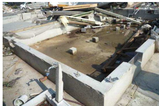
Fig. 7 Foundation of blown off wooden house ( quote from the report of KAKENHI, 2013 )
