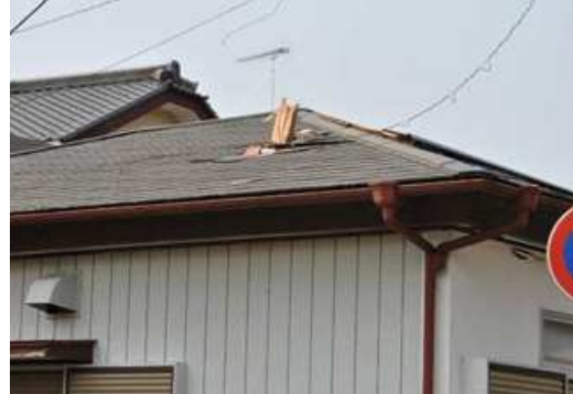
f. Timber stuck into a roof
