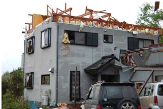
Fig. 12 Blown off roof ( quote from the report of KAKENHI, 2013 )
