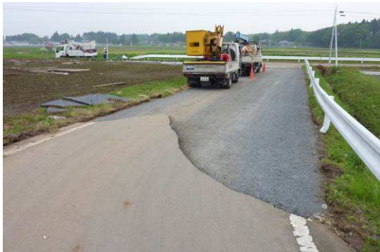
a. Exfoliation of asphalt
