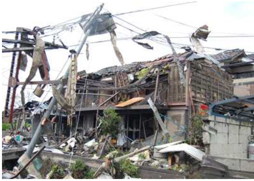
a. Flying debris twining around power lines
