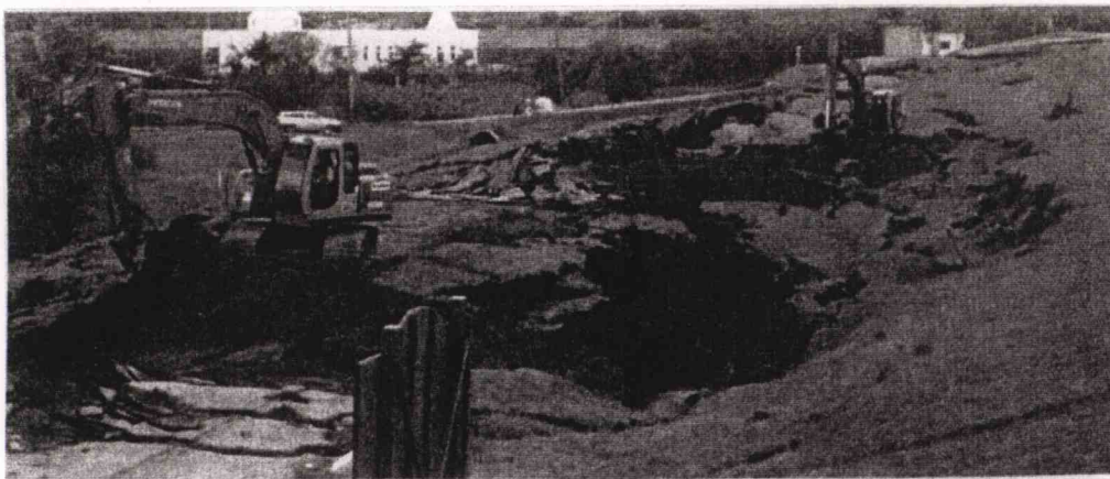
Photo 1 Damage of river bank due to liquefaction at the Tokachi river
