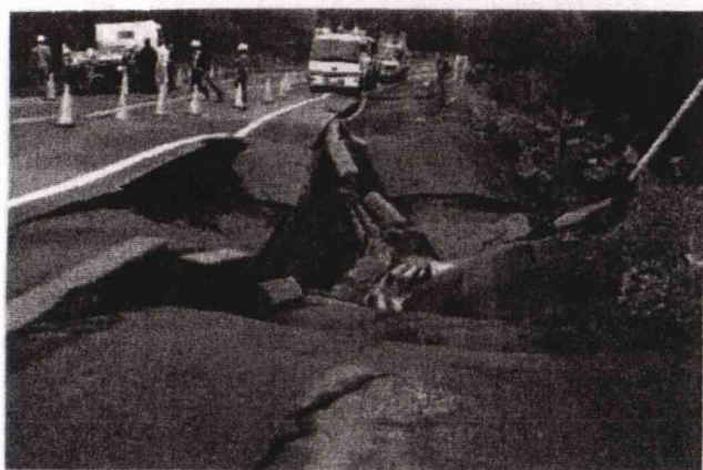
Photo 2 Damage of road
