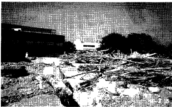
Photo 7 Sediment and driftwood deposited at the school building. The reinforced concrete building was buried one floor deep with sediment (taken at the place of ③)
