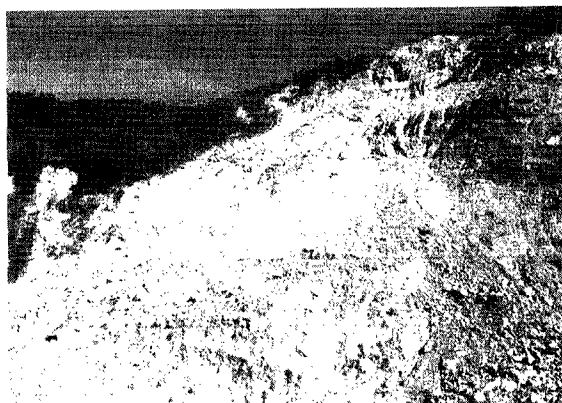
Photo 16 An example of the landslide presumably along the bedding plane (in the mountains to the east of the Qingshui-shi River).
