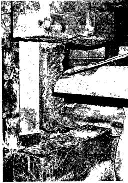
Photo 5 Repair detail observed at Warner Center Plaza #3
