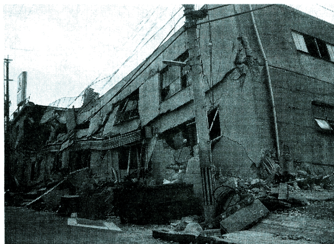
Photo 19 Collapse of a factory building.
