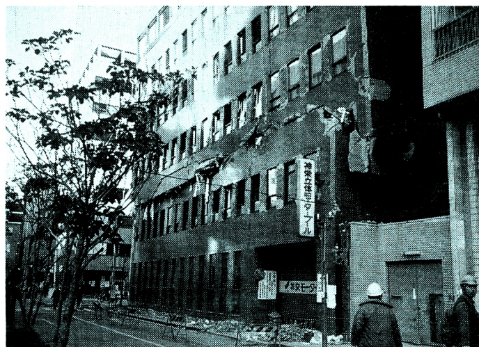
Photo 14 7-story building with a collapsed 3rd story.
