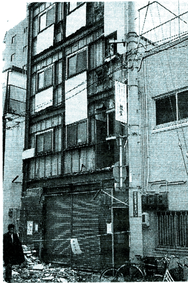
Photo 22 Steel structure with loss of cladding.
