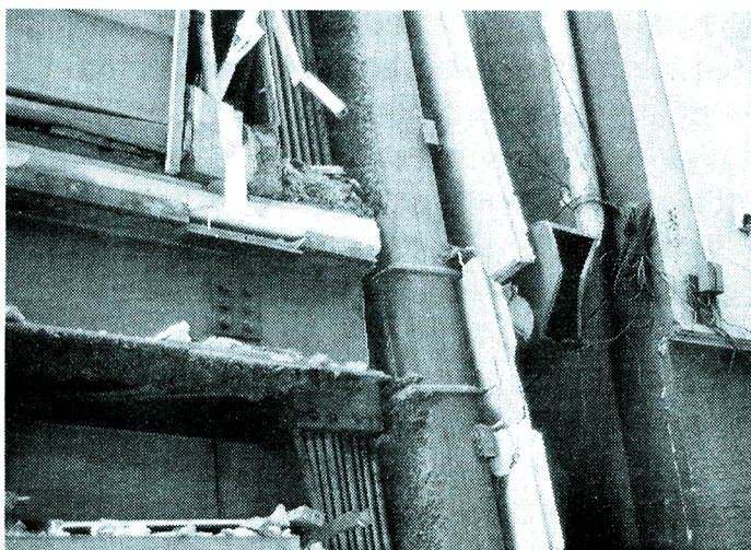
Photo 28 Failure of welded part at the beam end.
