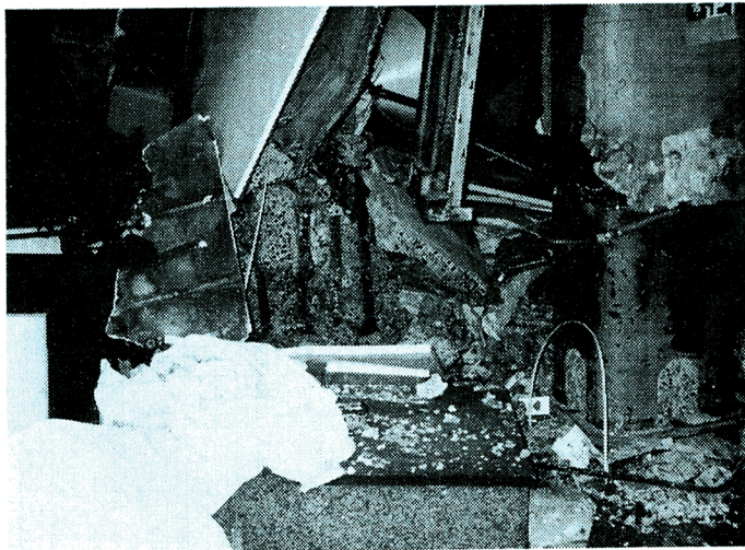
Photo 26 Failure of anchor bolts.
