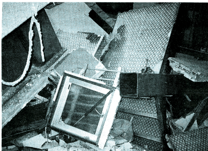
Photo 27 Failure at the top of column.
