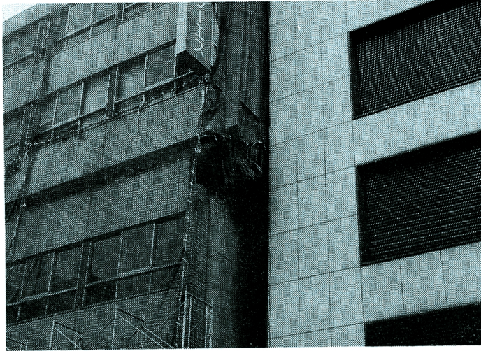
Photo 15 6-story building with a collapsed 4th story.
