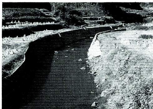
Photo. 2. Reventments damage in the Takimizu River.
