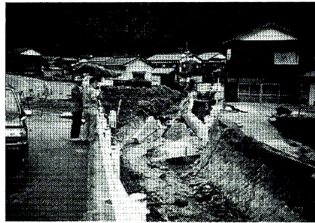
Photo. 3. Failure of revetments in the Satu river.
