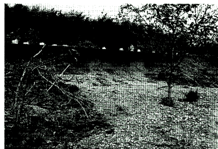
Photo. 11. Slip failure of the interior slope of levee near the station of Haemi bridge. (Photo by Notogawa Town Office)
