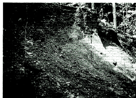
Photo. 12. The downstream slope of the breach shown in Photo. 7.
