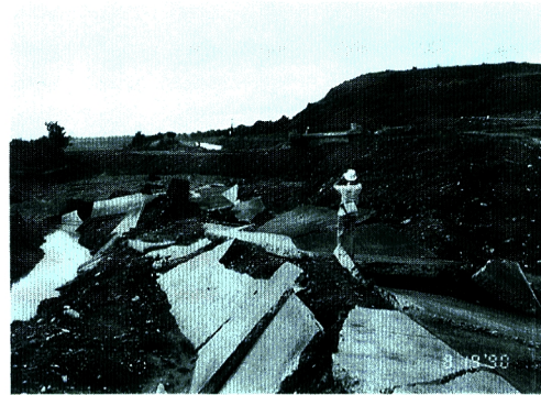
Photo 19 Damage to the road at St. Monica bridge.
