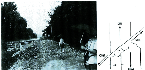
Photo 16 A surface faulting at Digdig (182 km from Manira).
