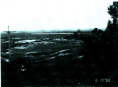
Photo 18 Damage to the embankment of irrigation ditch beside St. Monica bridge.
