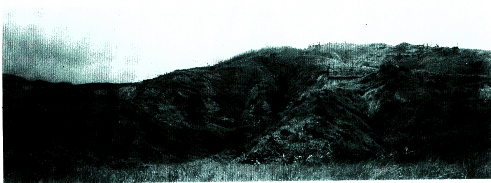
Photo 22 Slope failure ridge at Baterya.
