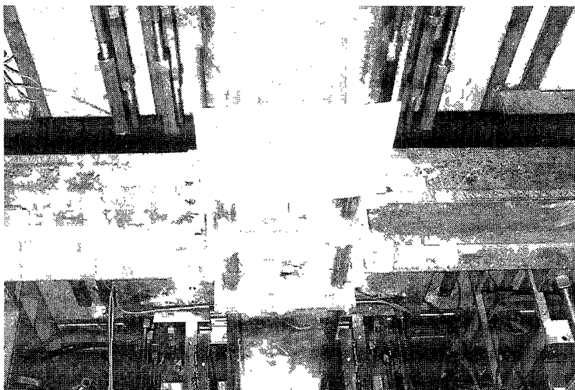
Photo 4 Fractured connection (conventional type)
