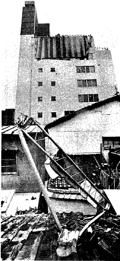
Photo. 12 Tent frame blown-away from the top of a 8-streedy building, KYOTO (by the courtesy of the Kyoto Shimbun).
