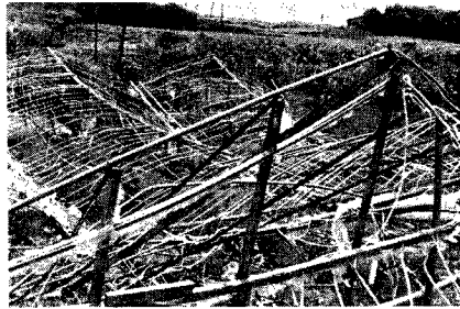
Photo. 4 Collapse of green houses with aluminum pipe frame, Gushikami, OKINAWA.
