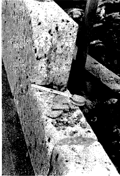
Photo. 8 Collapse of a block fence.
