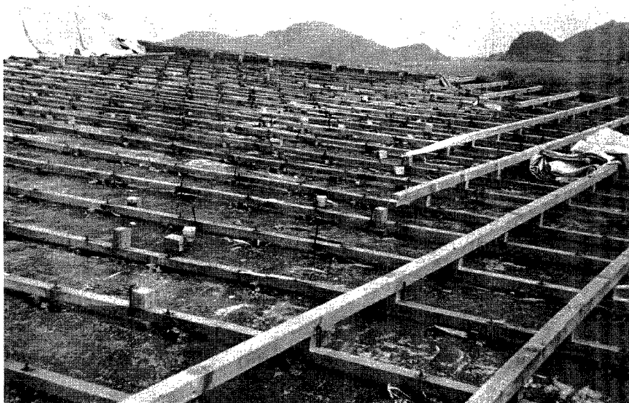
Photo. 2 Ruin of the blown away roof of Ōmi Plaza Hotel.
