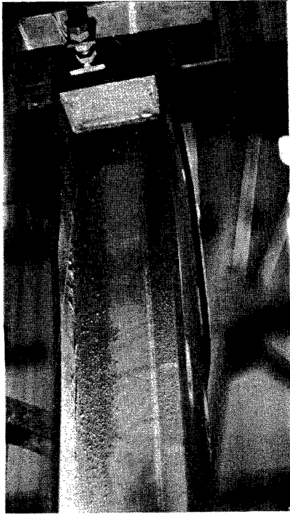
Photo. 8 Local buckling of column top (BC5).
