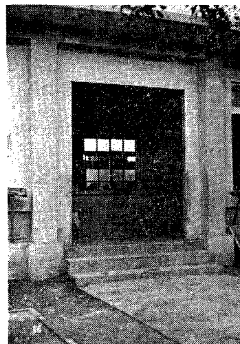
Photo. 4 A damage of reinforced concrete building; wreckage of a door.
