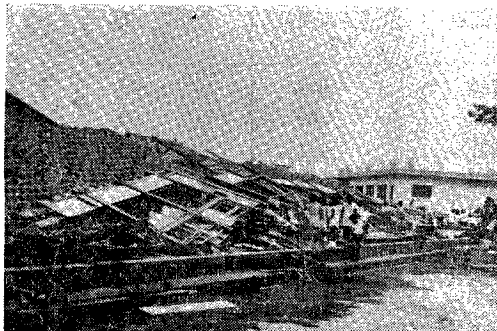
Photo. 2 Collapse of a wooden school-building.
