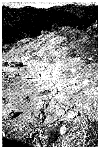
Photo. 3 Crack occurred in the neighbourhood of Shaft 1.
