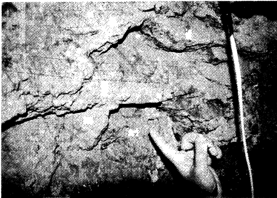
Fig.7 Photos of the gently dipping fault (potential sliding surface) found in the lower tunnel.
