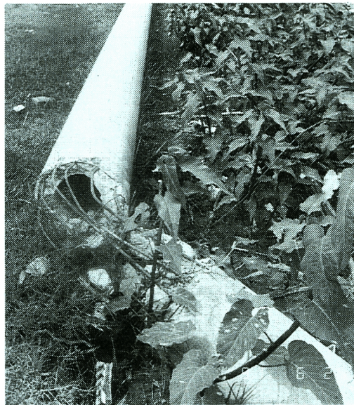
Photo 3. Broken electric line pole.
