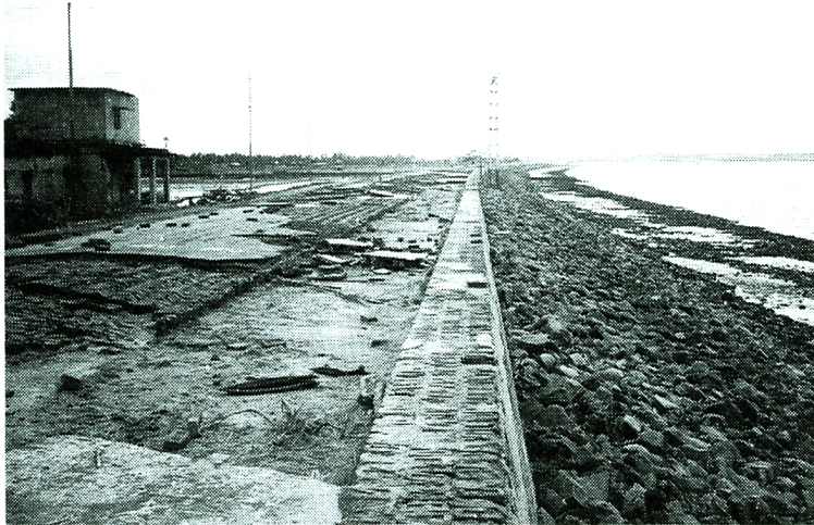
Photo 7. Damaged levee that had been armored with asphalt and bricks along the right side of the mouth of the Karnafuli River.
