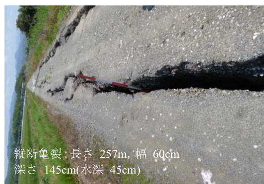
図-6 縦断亀裂 (矢形川右岸,浮島橋上流 1)
