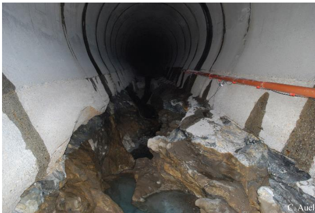
Fig. 1 Invert abrasion of Palagnedra bypass tunnel, Ticino, Switzerland (Auel 2014)
