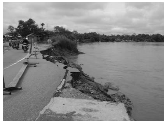
Fig. 2 Collapse of river banks at Sesayap River, Malinau, East Kalimantan, Indonesia
